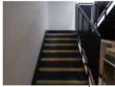
Further handrail on wall side recommended.
